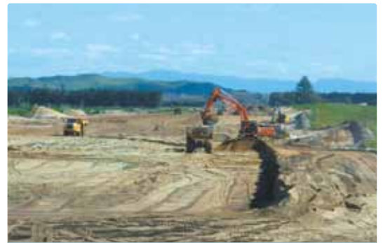
One of many areas the public won't see until the highway opens in 2016. The 'sand cut' is located between Parton Road and Kaituna River.
