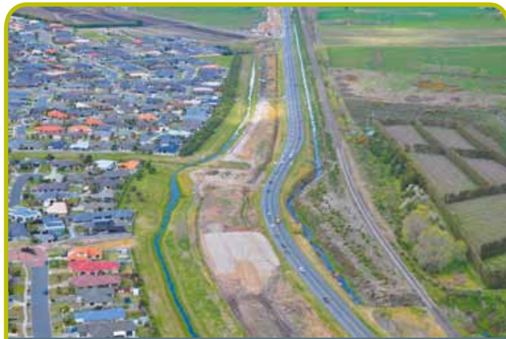
1 SH2 - trial embankment at the Maranui Swale, Bruce Road top left hand corner
